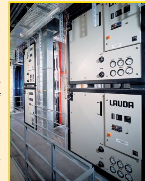
Modular construction of heat transfer fluid systems. The picture shows the new production site at ALTANA, Singen, Germany
