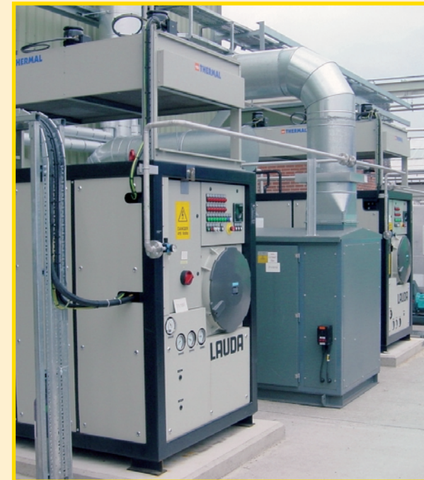
The two LAUDA process cooling units installed outside. Chilling unit with temperature range from -80 up to 140 °C at the front.
