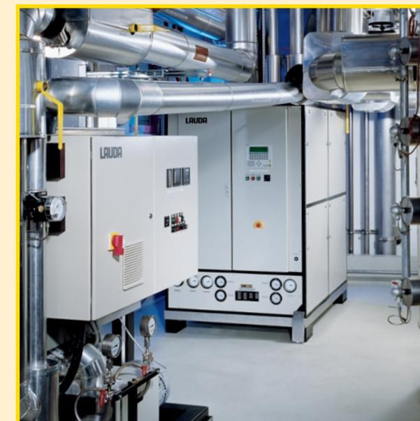
Modular plant for temperature control made by LAUDA; coupling of heat transfer system with process cooling unit Operating range from -40 up to 200 °C Pressure reaction centre at Merck KGaA/Darmstadt
