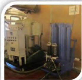
Petrochem Air Compressor China
