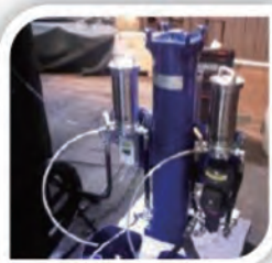
Petrochem Plant Compressor USA
