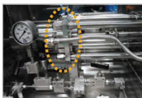
Cooling line on high pressure part 高压泵体冷却装置
