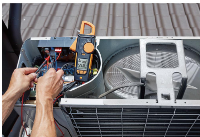
测量空调外机电压
