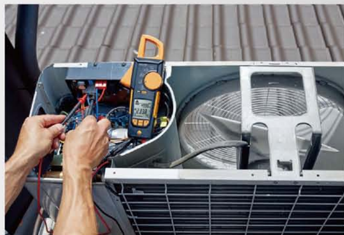
测量空调外机电压
