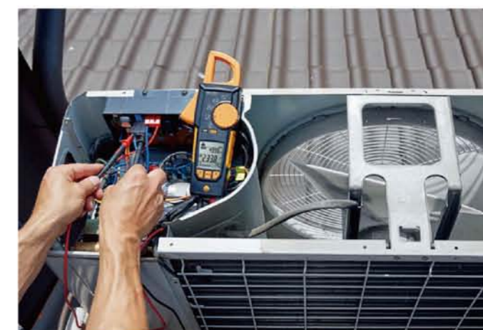
测量空调外机电压
