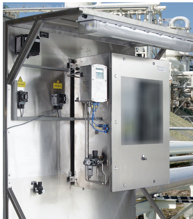
Image: example of EnviroLyzer® in an ex-proof cabinet at a LNG terminal.
